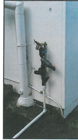
Headworks of the new irrigation system incorporating filter, solenoid and pressure reducing valve
